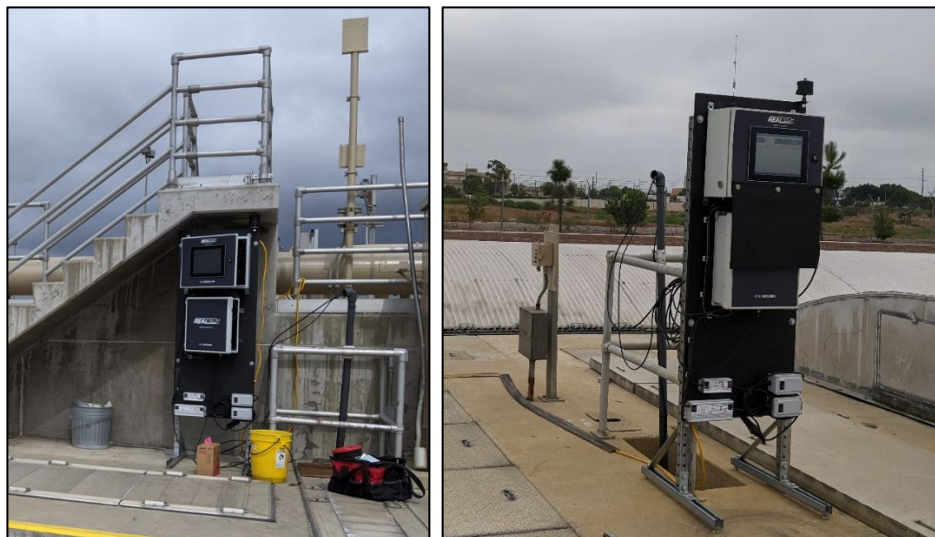
Figure 3-23. Real Tech in Primary Effluent (left) and Secondary Effluent (right) at JWPCP.
