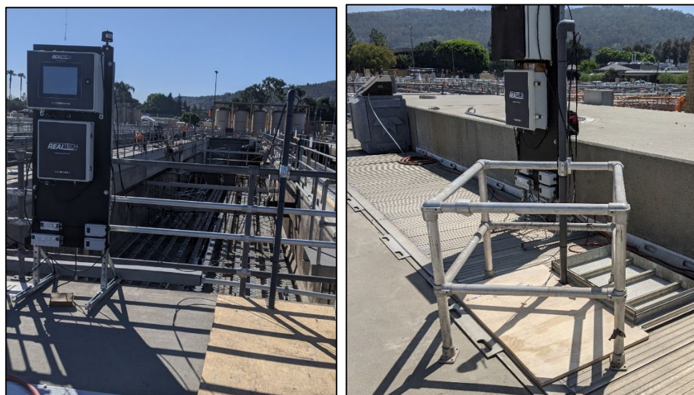
Figure 3-24. Real Tech in Primary Effluent at SJCEWRP.
