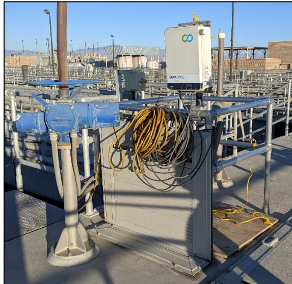
Figure 3-28. Sentry Probe in LANWRP Primary Effluent.
