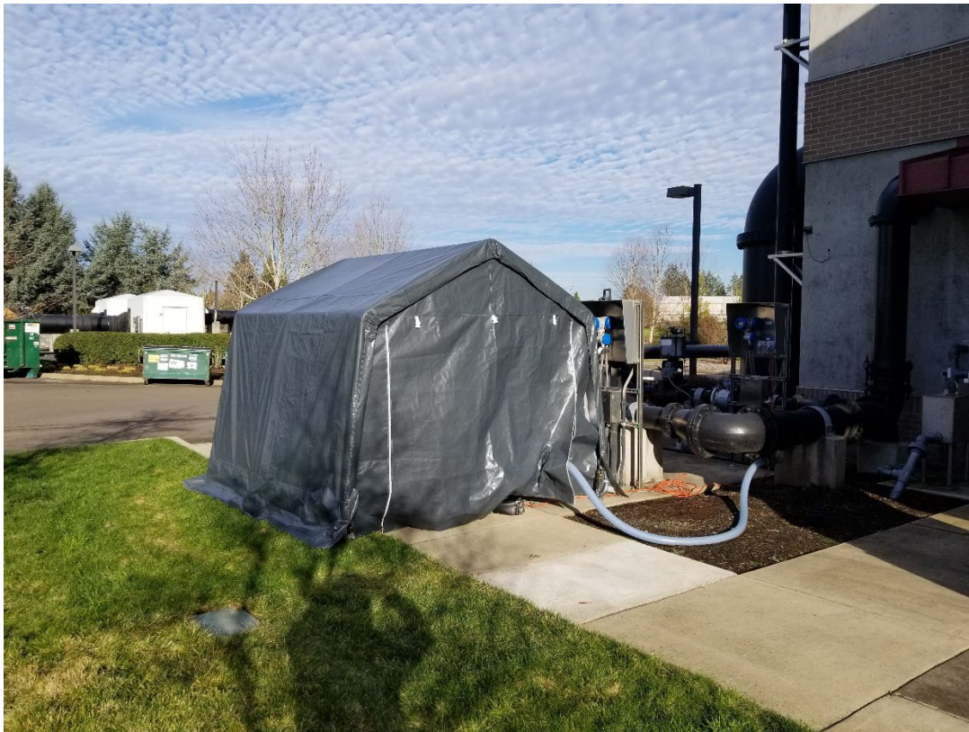
Figure A-1. Flume located at the Forest Grove WWRF.
