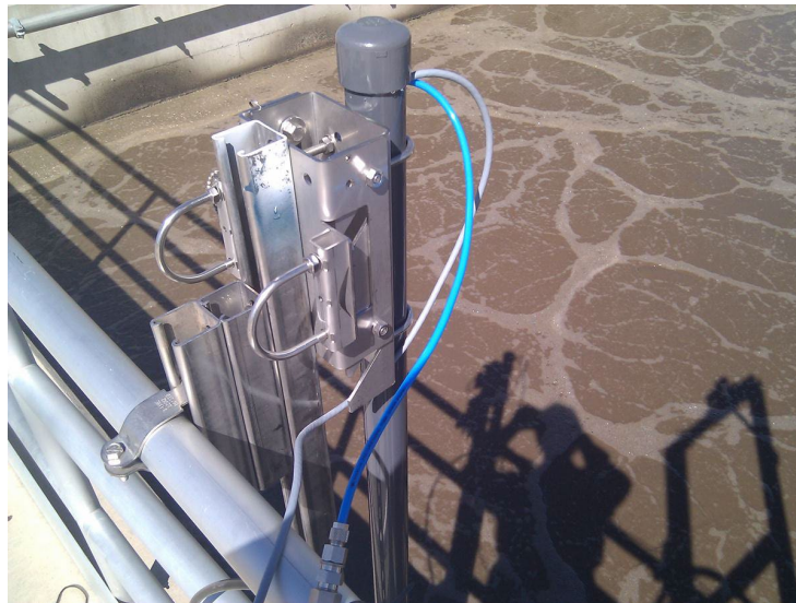
Figure 2-5. Ammonia sensor installed at the Aeration Basin Site (City of Phoenix).
