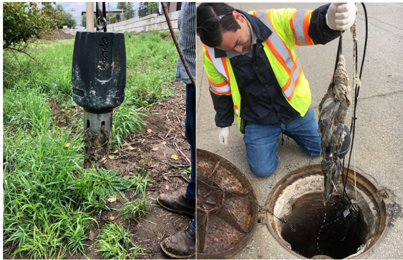
Figure 5-2. Ragging of the Sensor Probes and Connective Wiring.
