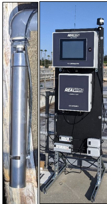
Figure 3-22. Real Tech Sensor (right) and Communication Unit (left).
