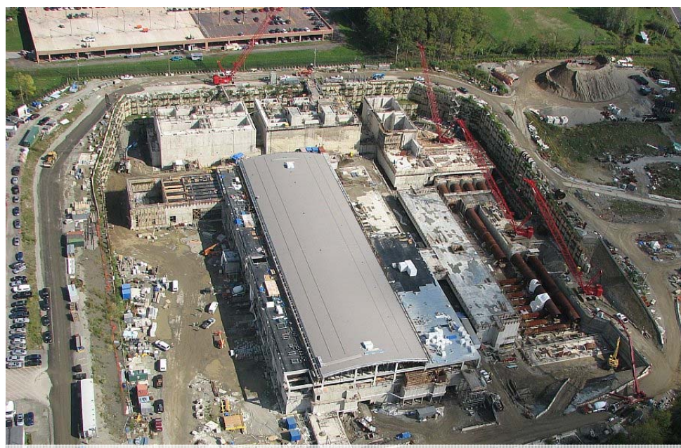
Cat-Del UV Disinfection Facility ($1.6 B)
