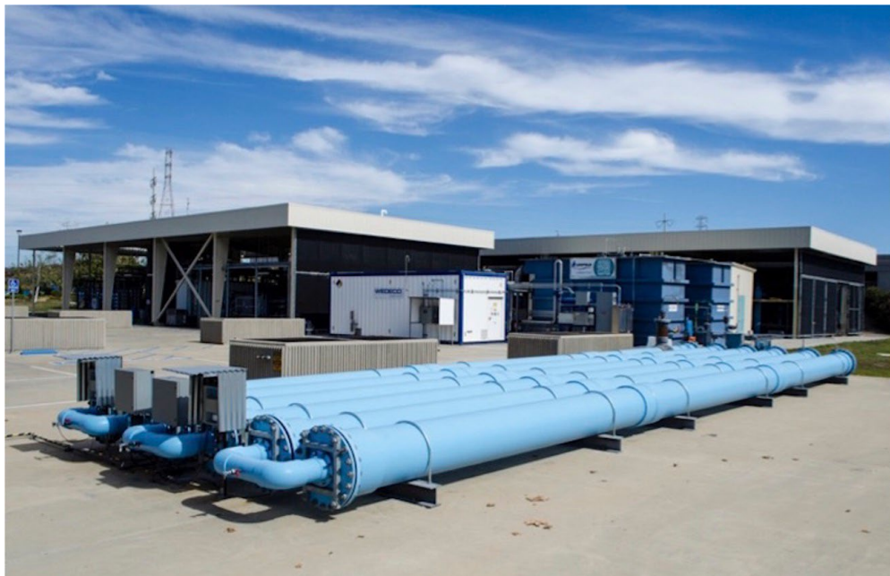
Figure 4-2. Ozone Pipeline Contactor at NCPWDF.
