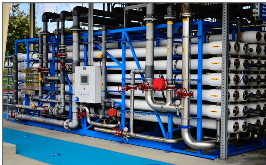
Figure 4-4. RO Skid at NCPWDF.
