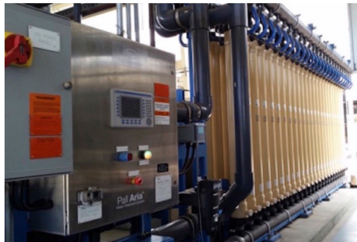
Figure 4-3. Membrane Filtration Skid at NCPWDF.
